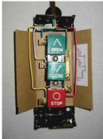
Photo #33 (NEMA-1 Station Wiring)
