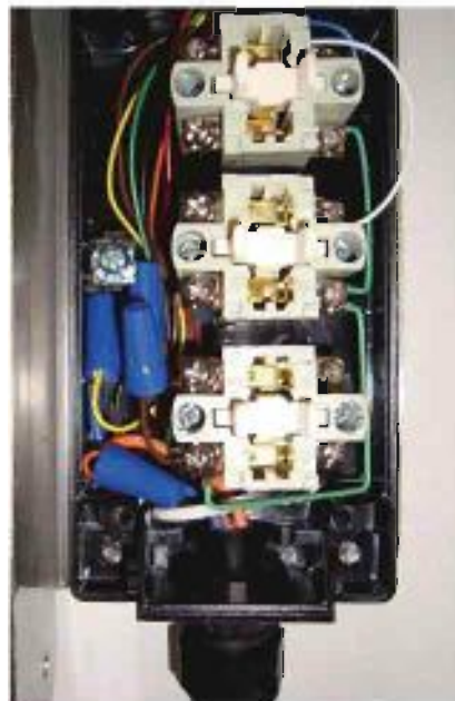
Photo #23 (NEMA 4 Wire Dressing)
