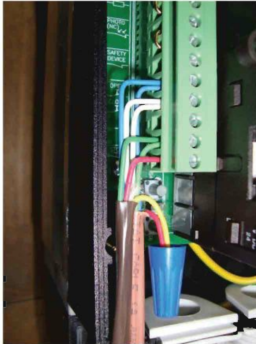
Photo #34 (Additional Station Operator Wiring)
