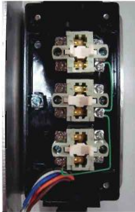
Photo #19 (NEMA-4 Common Wiring)
