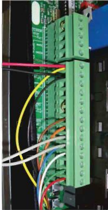
Photo #39 (RF Receiver Wiring)
