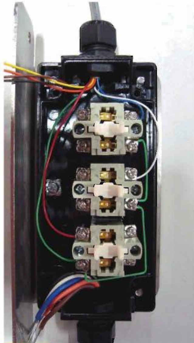
Photo #21 (NEMA 4 Control Wiring)
