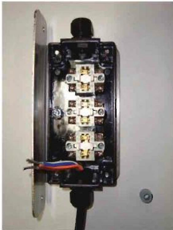
Photo #18 (Photo Eye Wire Routing)
