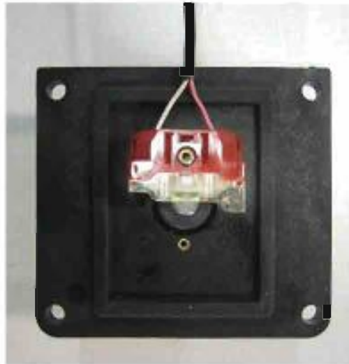
Photo #37 (Pullcord Switch Station Wiring)
