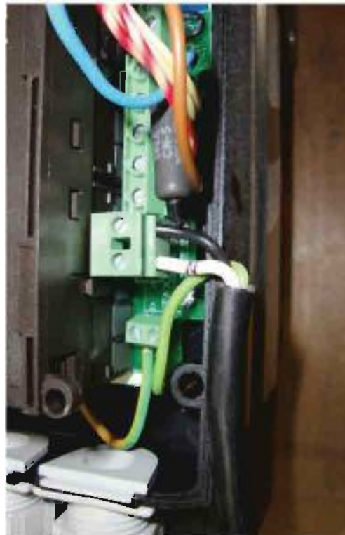
Photo #17 (115VAC Power Wiring)
