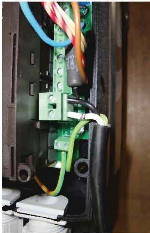
Photo #17 (115VAC Power Wiring)
