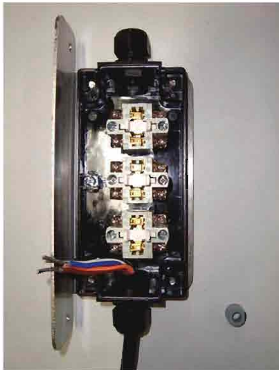
Photo #18 (Photo Eye Wire Routing)
