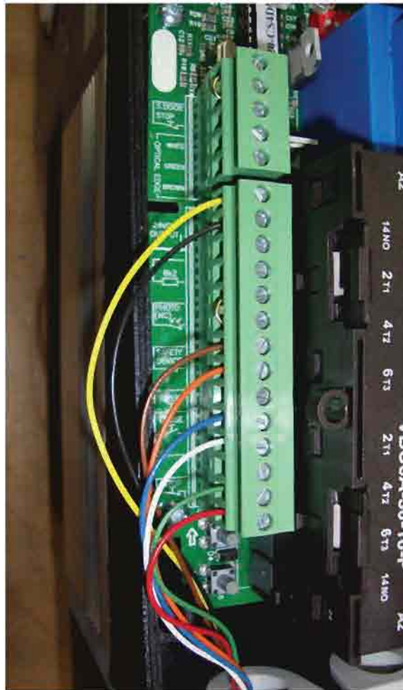
Photo #24 (Operator Low Voltage Wiring)
