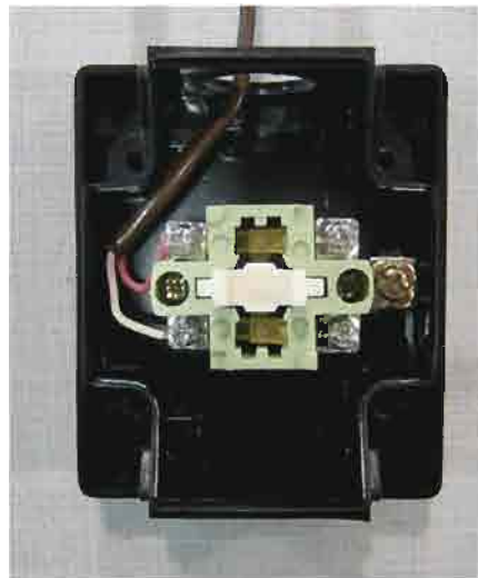
Photo #36 (Single Button Station Wiring)
