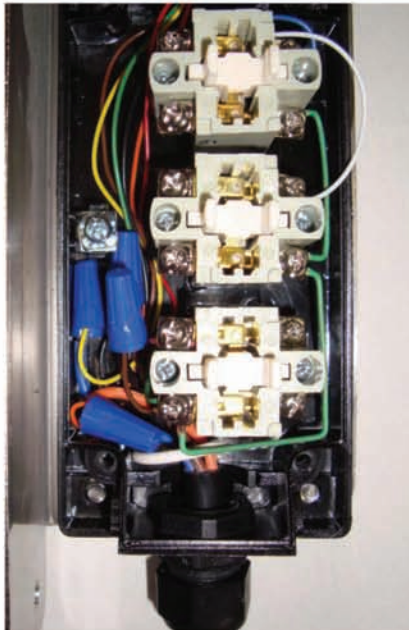
Photo #23 (NEMA 4 Wire Dressing)
