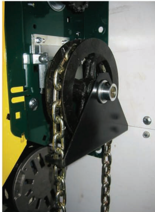
Photo #14 (Hoist Chain Routing)
