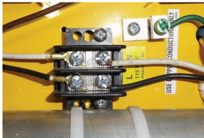
Photo #19 (Power Connections)
