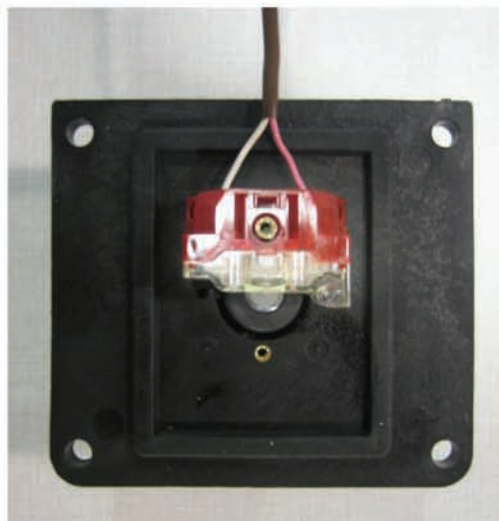
Photo #41 (Pullcord Switch Station Wiring)
