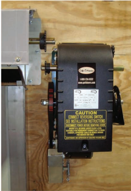
Photo #9 (External Operator Mounting)
