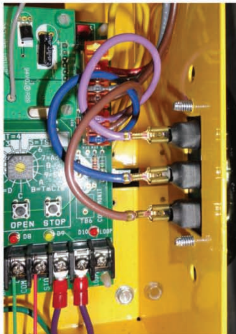
Photo #33 (RF Receiver Wiring Swap)
